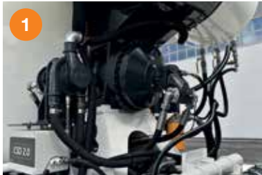
Hydraulic water pump.
